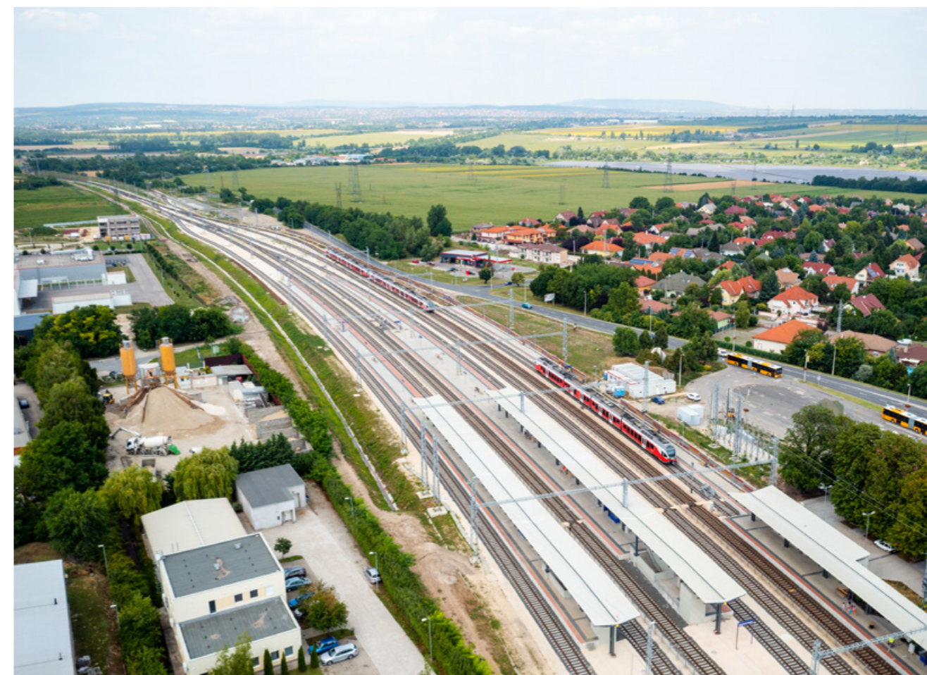
Reconstruction of the Százhalombatta – Pusztaszabolcs railway line and setting up the railway control system
